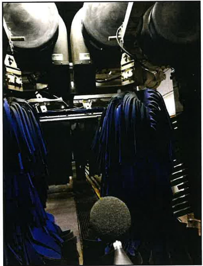
Photo 2. Dryer Blowers With Silencers
