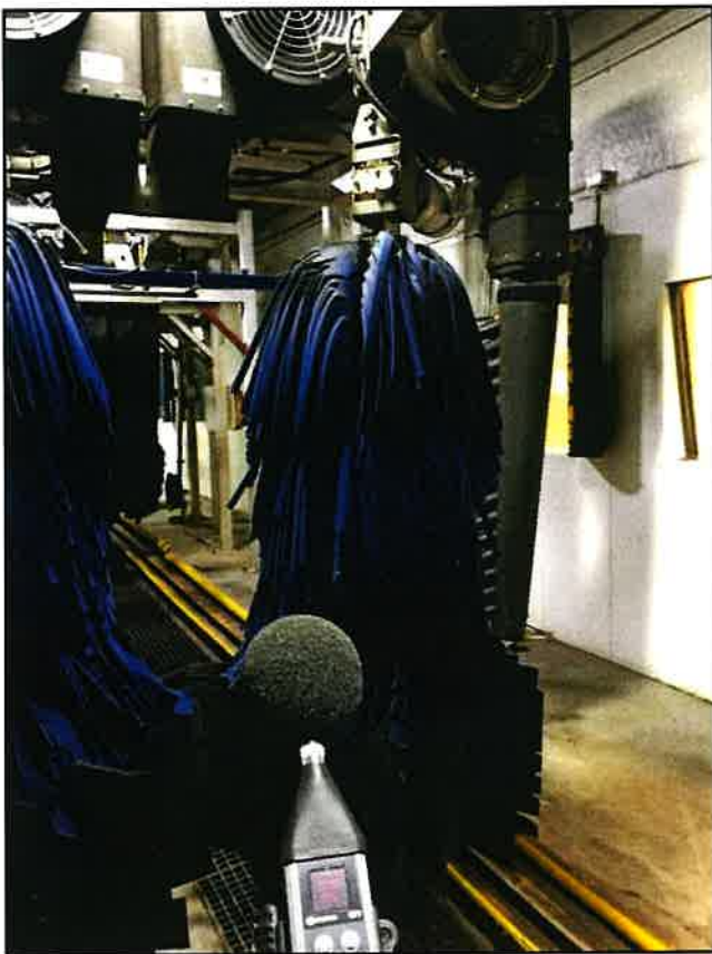
Photo 3. Dryer Blowers Without Silencers
