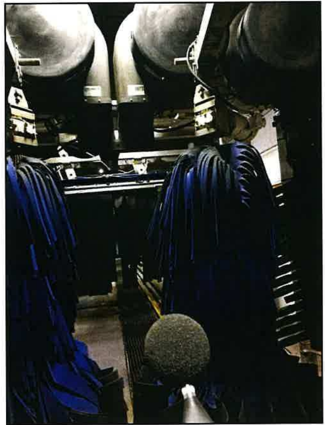
Photo 2. Dryer Blowers With Silencers
